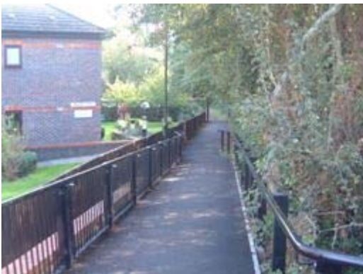
Steps on path replaced with an anti slip ramp to facilitate disabled access and three new lighting columns installed.
